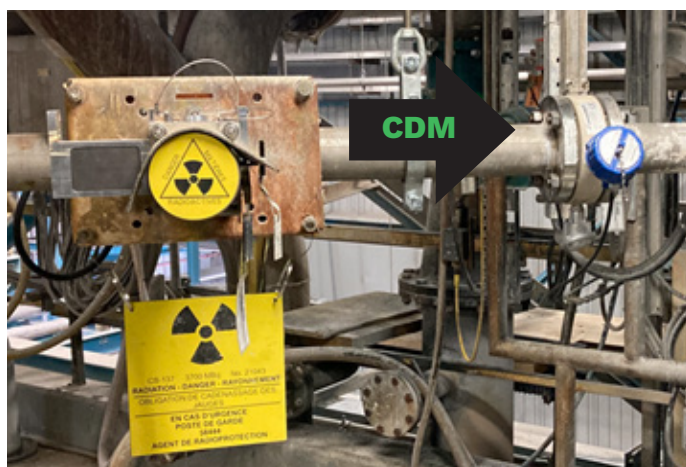
The CDM installed in the same line as to where the radiation-based density meter is measuring density
