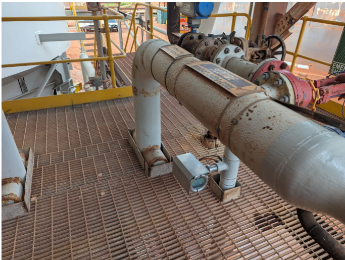
Fig. 1: The Rhosonics SDM installed at the Rio Tinto Gove site.
