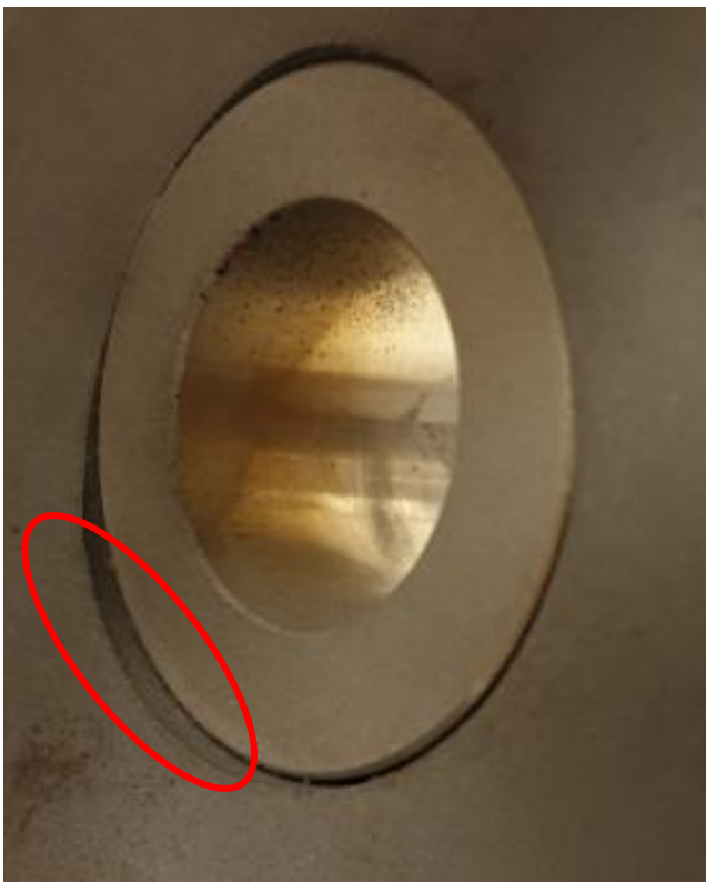
Uneven edges will always be visible on two sides of the weldolet inside the pipe due to the roundness of the pipe.
