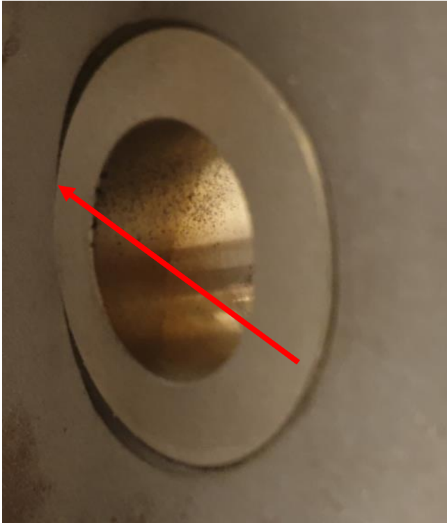
The arrow indicates the flow direction. The weldolet is perfectly flush.
